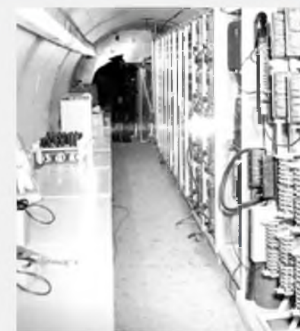
Data interception equipment stationed in the tunnel
